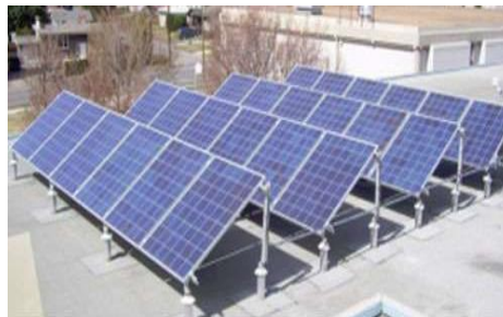
Figure 46 SOLAR SYSTEM ON ROOFTOP
