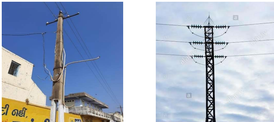
Figure 69 Concrete Pole and Lattice Steel Tower
